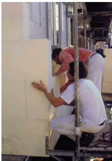
Fig. 1 – Fixing of PUR rigid foam blocks of 300 mm thickness in an ETICS system for a passive house
